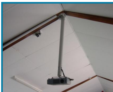
Ceiling mounted data projector
